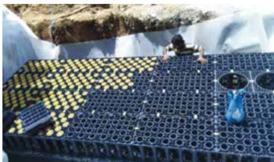
The rainwater collected by the pipelines will arrive at a tank where the water undergoes purification. (Photo by courtesy of RCEES)
